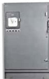
300 HP 600V Starter in Type 3 Enclosure
