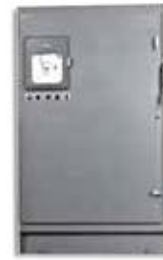
400 HP 600V Starter in Type 3 Enclosure
