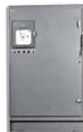
400 HP 600V Starter in Type 3 Enclosure
