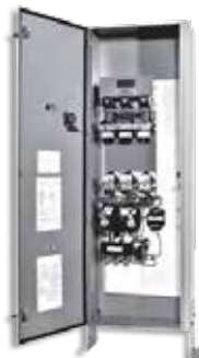
300 HP 460V Starter in Type 12 Enclosure
