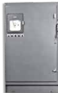
300 HP 600V Starter in Type 3 Enclosure
