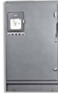
300 HP 600V Starter in Type 3 Enclosure
