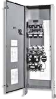
300 HP 460V Starter in Type 12 Enclosure
